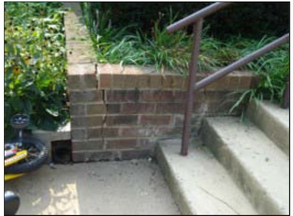
Photo #4. Brick Wall Damage
