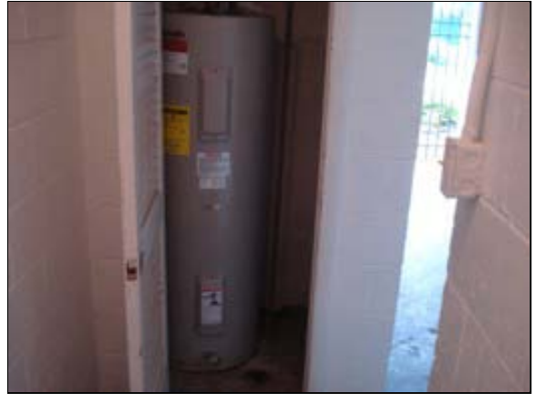
Photo #8. Water Heater
