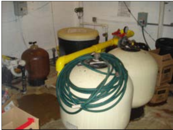
Photo #9. Pool Filters
