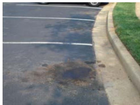
Stained Asphalt - Typical
